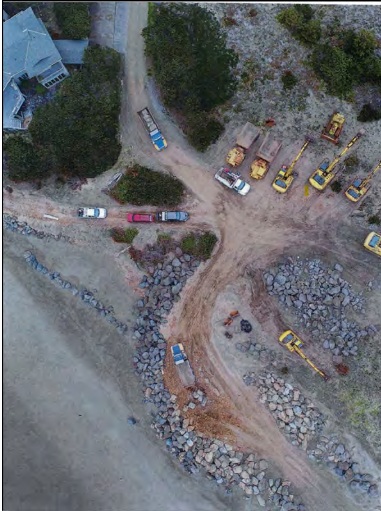
Figure 1: Aerial image of the northern portion of the Beach Grass Lane common area property, with improvements (grading, imported rock, slope stabilization, etc.) to allow construction equipment and emergency vehicle access to the Salishan Spit shoreline area (photo provided by client).
