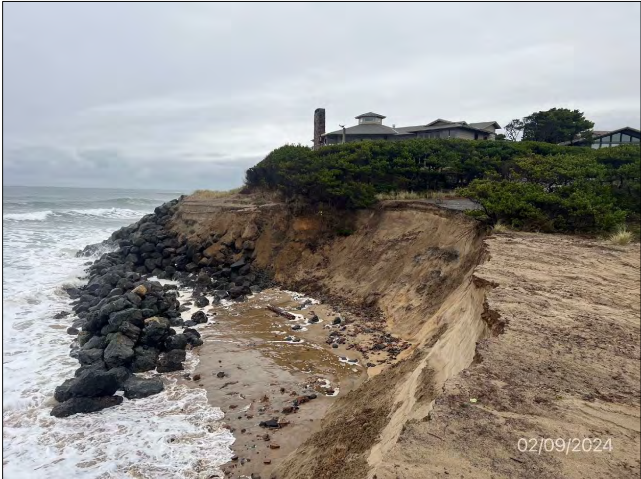
Photo 6: View of the erosion caused by the rip embayments in January and early February 2024, looking north, same location as Photo 4 (photo date: February 9, 2024).
