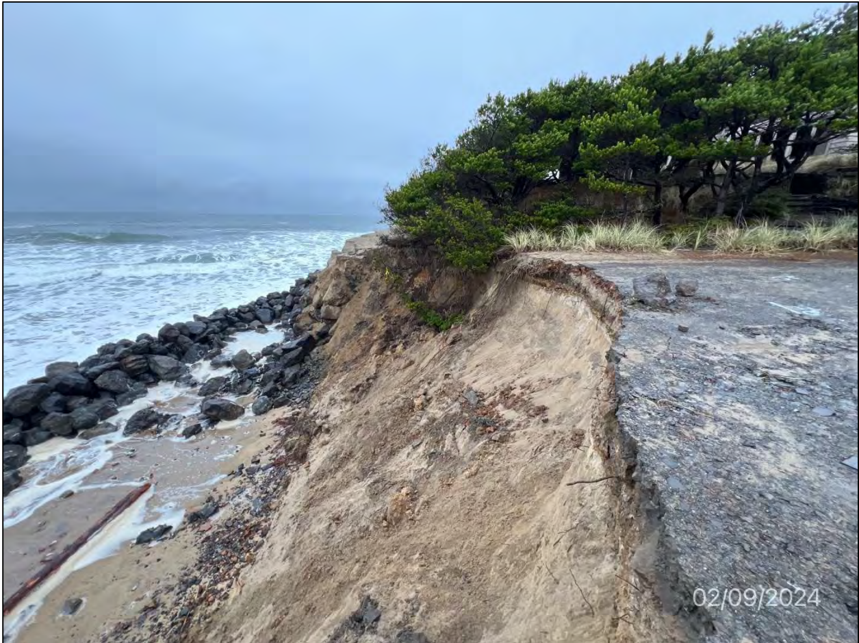
Photo 7: Beach Grass Lane roadway subject to erosion in early February, looking north (photo date: February 9, 2024).
