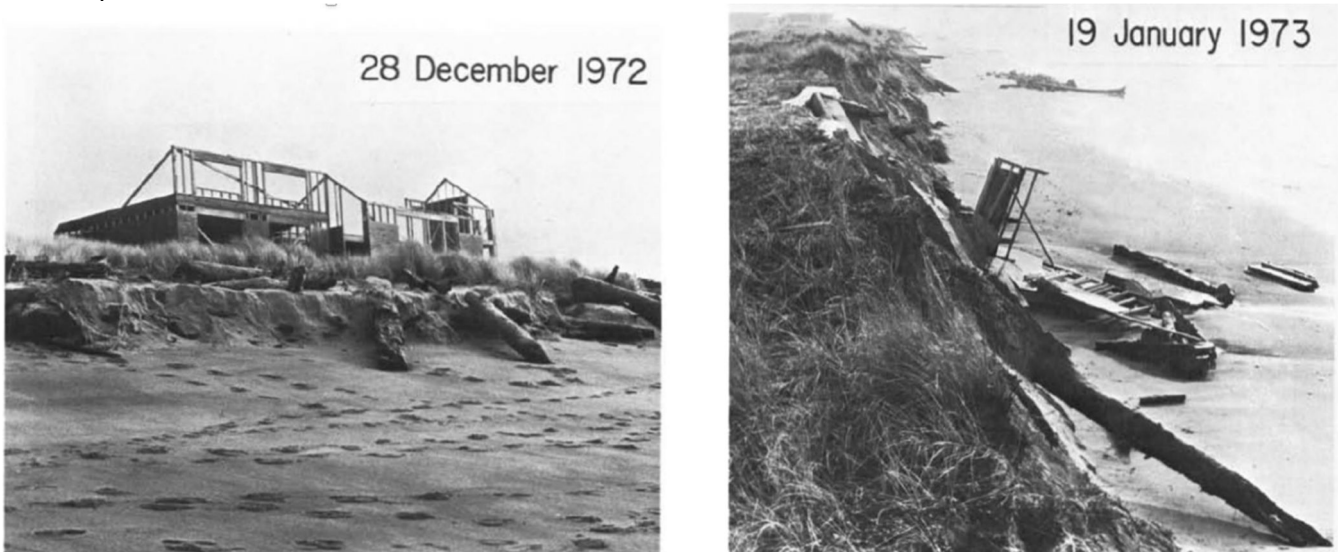
Photo 1: Erosion and destruction of the house under construction on lot 226 of Salishan Spit. From Komar and Rea (1976)
