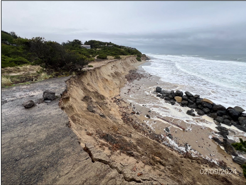
Photo 1: Looking south from Beach Grass Place across beach frontage of Beach Grass Lane common area. Older temporary rip-rap placed can be seen on the right side of the photo.
