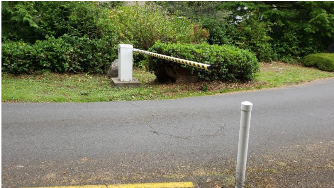
General Site - Entry Gate, Maintain & Repair
