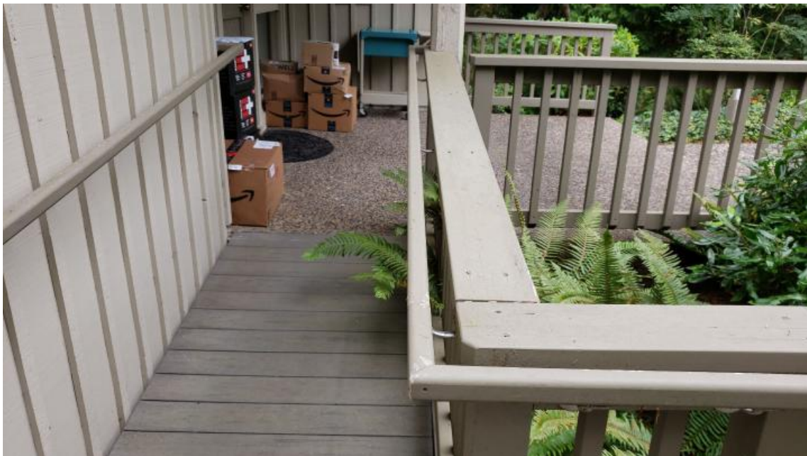
Building Exterior - Deck Surface, Wood Decking [Replace]
