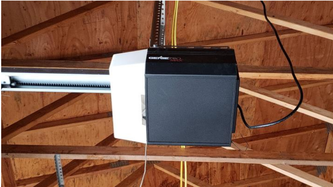
Building Exterior - Garage Door, Operator
